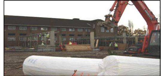
Front view of dining hall - very large windows will be installed between the three large upright columns
